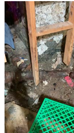
717 HoseBibb Leak LaundryRoom2559.MOV
